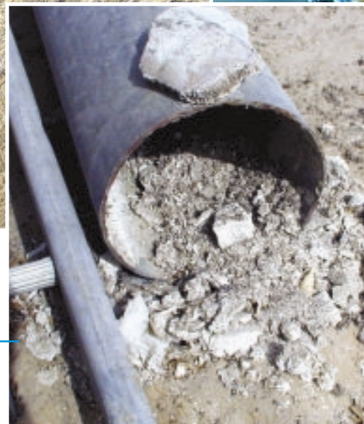
Deposits of CaSO 4 in a sludge pipe
